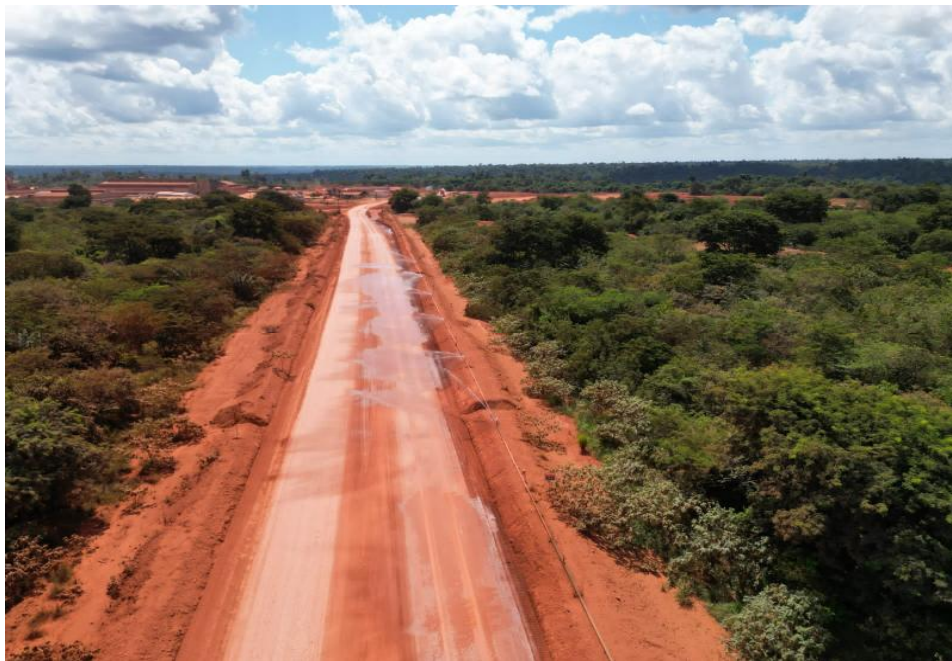
Figure 4. Automatic water sprinkler system for dust control
